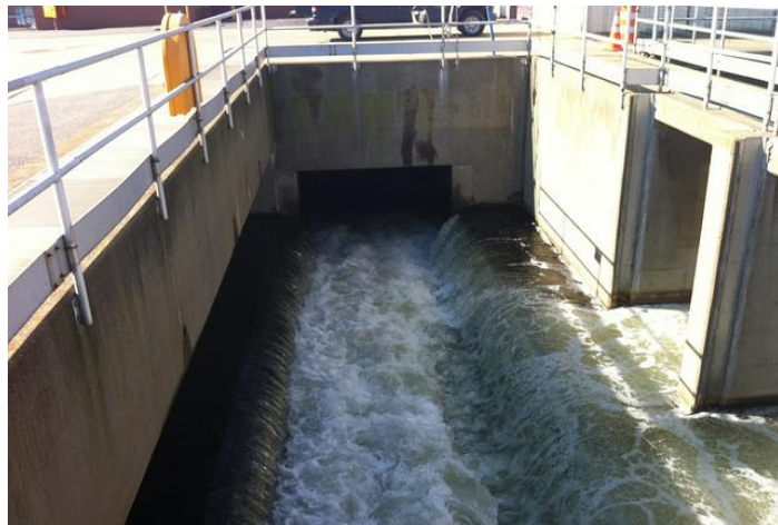
Wastewater discharge into the Ohio River near Pittsburgh. Photo courtesy of WESA.
