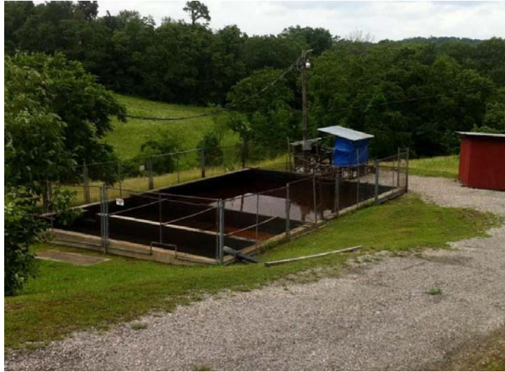
Storage pit at the Ginsburg injection well, Ohio. Photo courtesy of Athens County Fracking Action Network.
