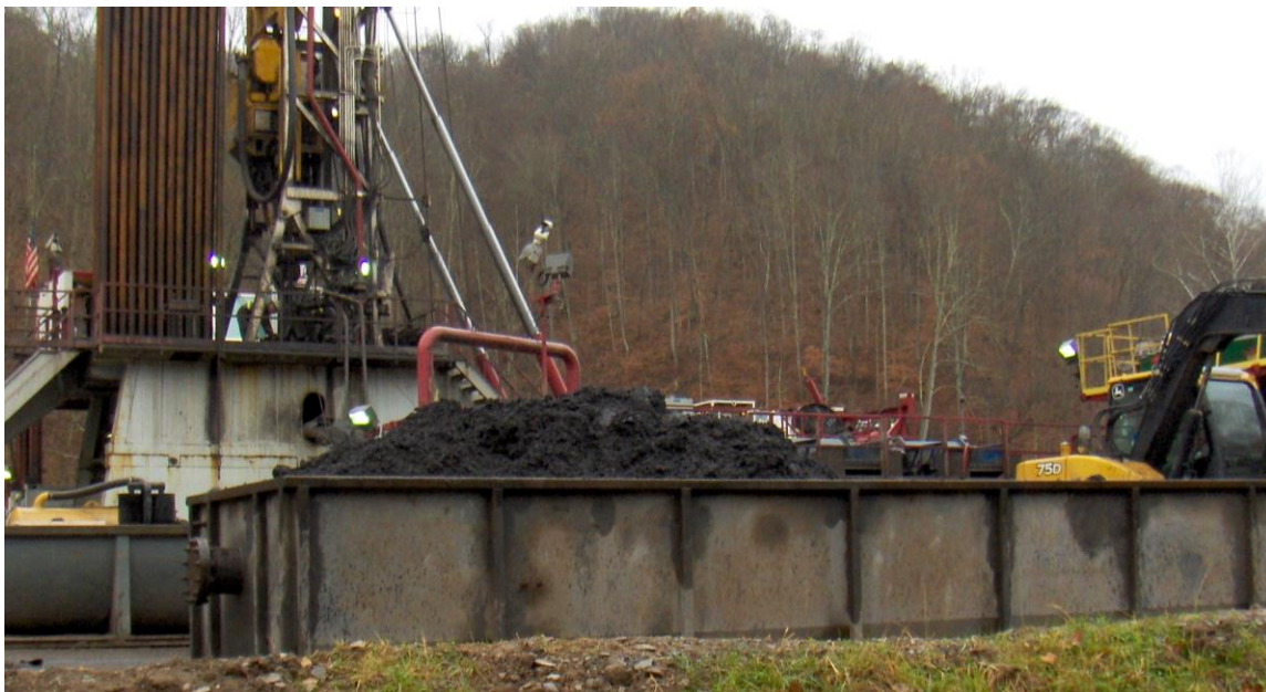
Drill cuttings stored at a well site in West Virginia. Photo by Bill Hughes.
