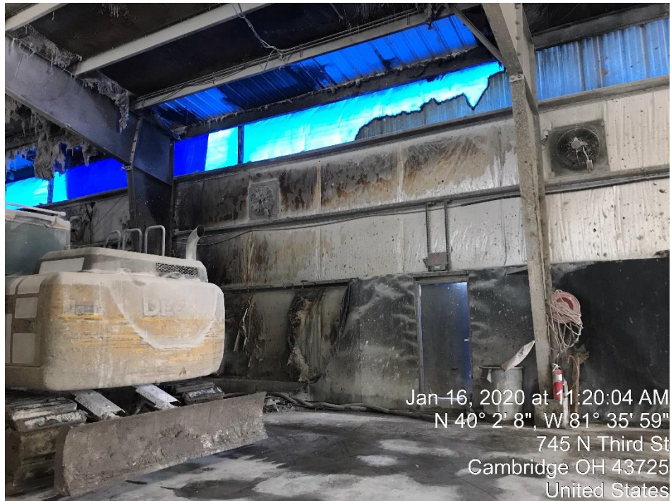
Building damage from fire
