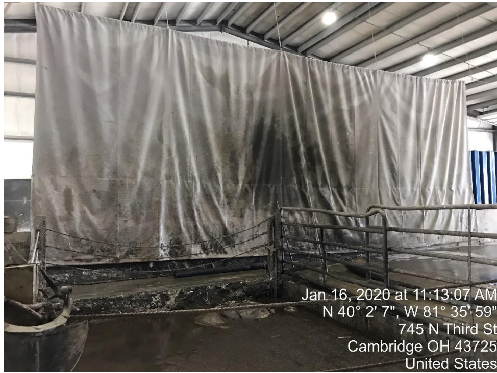
Industrial processing area curtain
