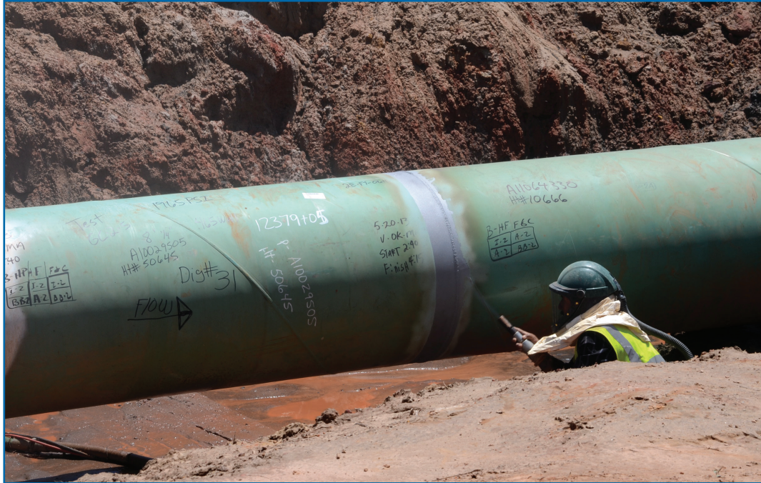
Workers in a trench are finishing the new replacement of pipe on a landowner's property.
