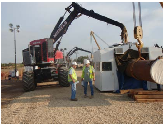
Figure 20: Automatic Welding Shack
