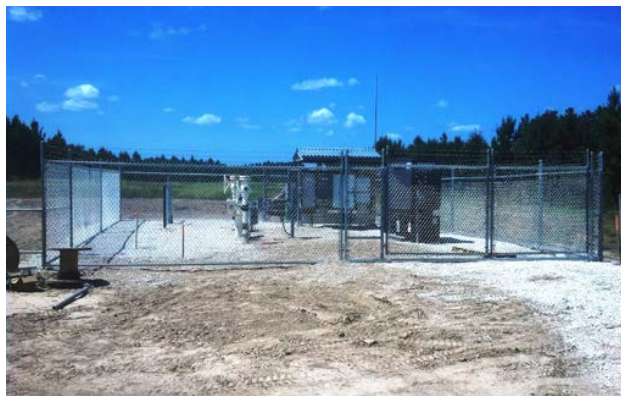
Figure 18: Typical Fencing around Valve site
