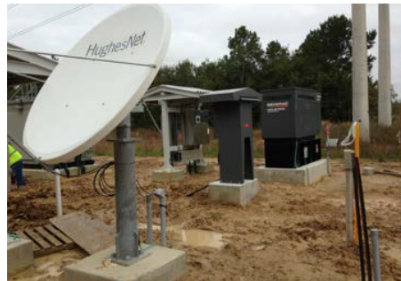
Figure 14: Remote Operation Equipment at Valve site.
