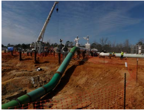
Figure 16: Valve at Pump Station
