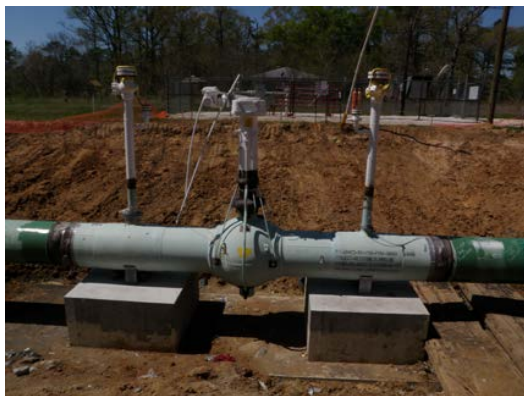
Figure 17: Concrete Pads for Valves.
