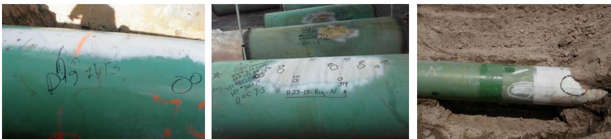
Figure 32, 33, 34 Examples of dents found with inspection tool.
