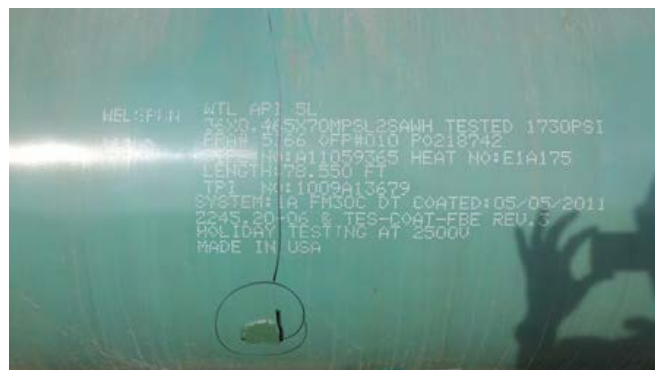
Figure 2: Pipe Specification Markings
