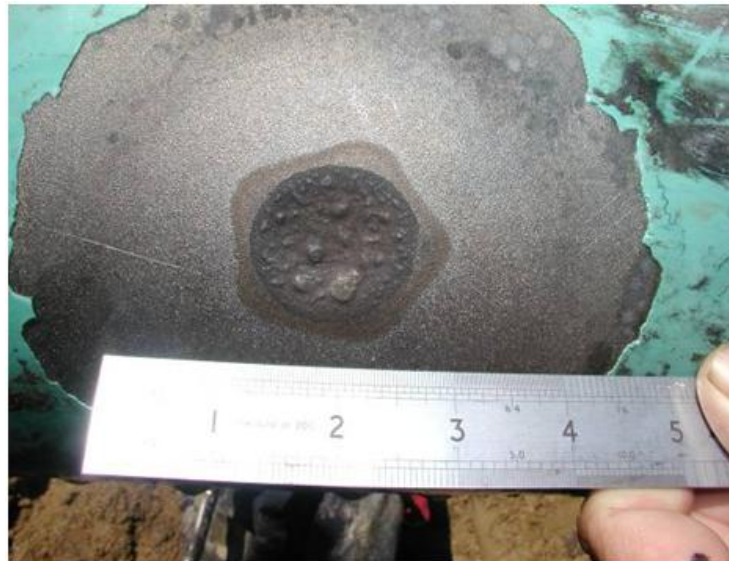
Figure 6. Typical A-C Corrosion Morphology
