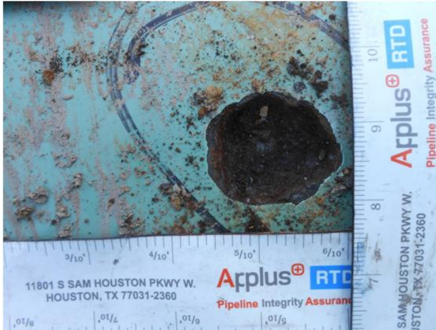
Figure 13. MP 996.33 –External Corrosion Pitting
