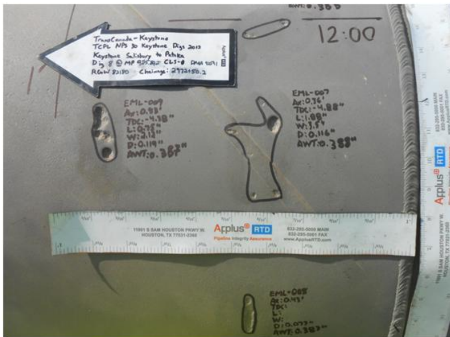
Figure 22. MP 925.89 – External Corrosion
