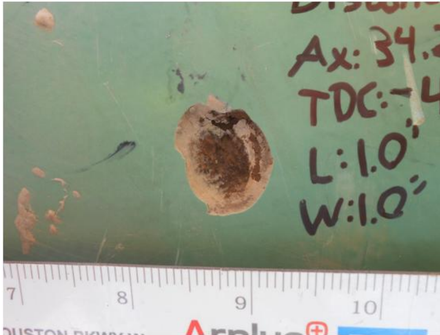
Figure 16. MP 1000.38 –External Corrosion Pitting
