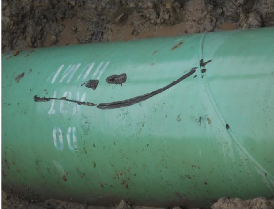
Figure 17. MP 997.67 –External Corrosion at Areas of Coating Damage
