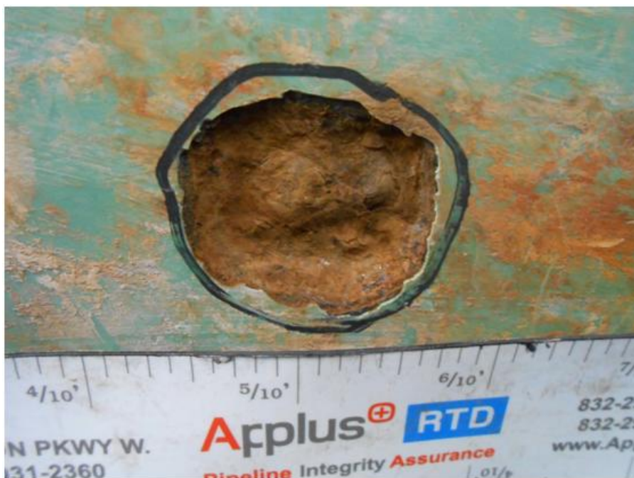
Figure 26. MP1000.32 – External Corrosion Pitting
