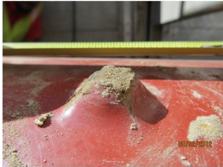
Figure 8. A-C Corrosion – FBE Coating “lift-off” and Cracking
