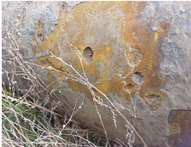
Figure 5. Typical D-C Stray Current Corrosion Morphology
