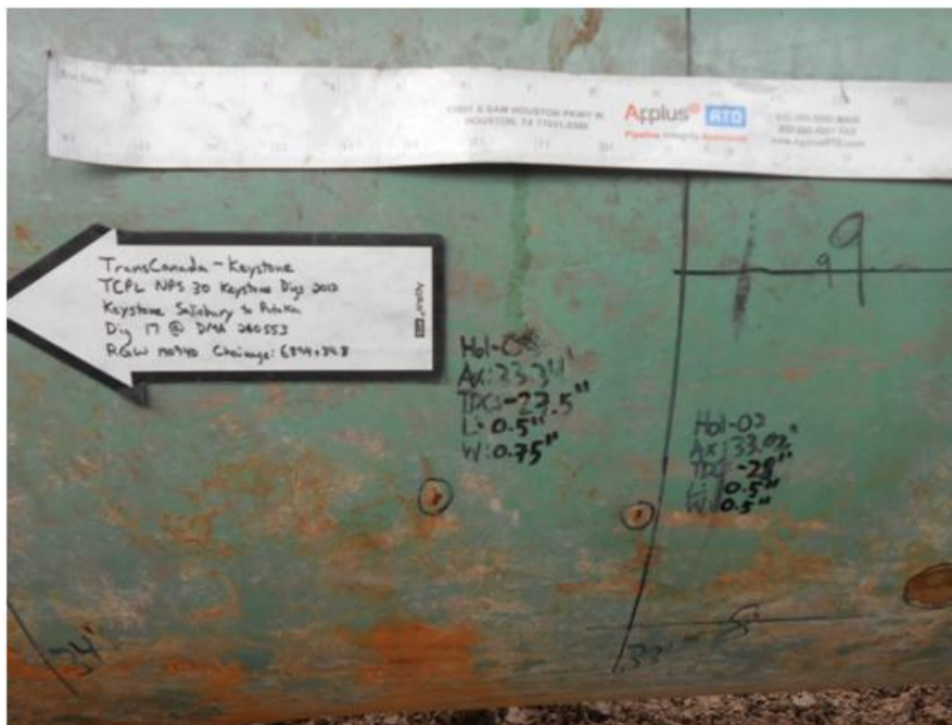
Figure 25. MP1000.32 – External Corrosion Pitting
