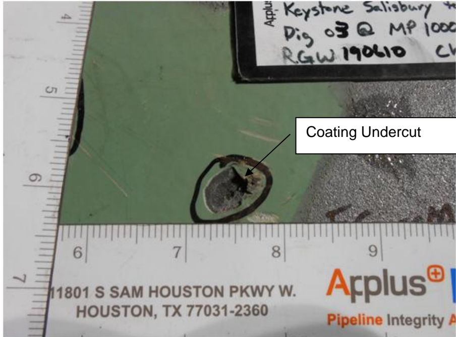
Figure 14. MP 1000.08 –External Corrosion Pitting
