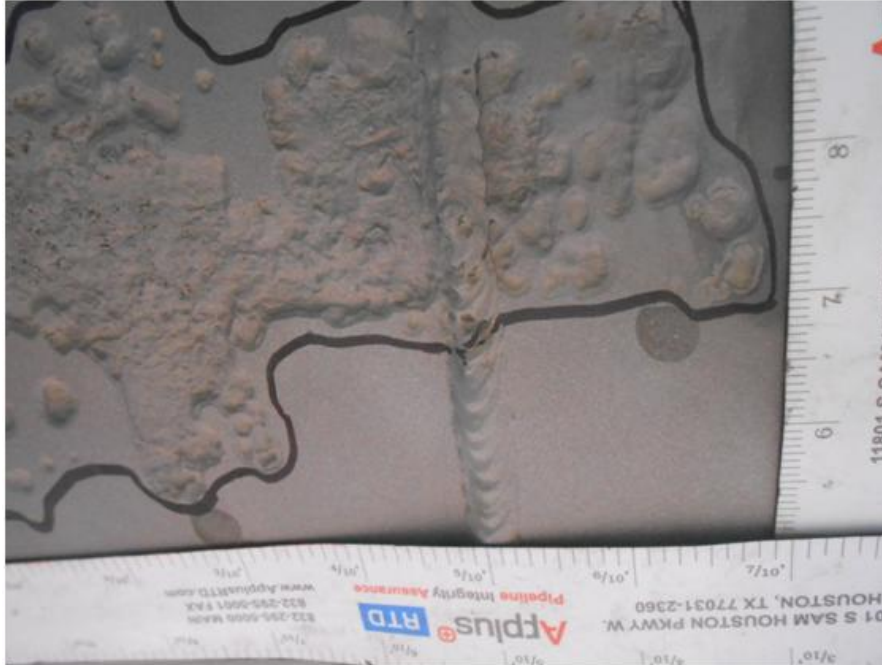
Figure 24. MP 999.97 – External Corrosion
