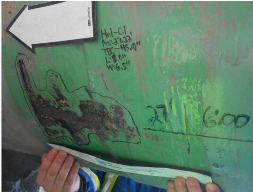
Figure 23. MP 999.97 – Coating Damage
