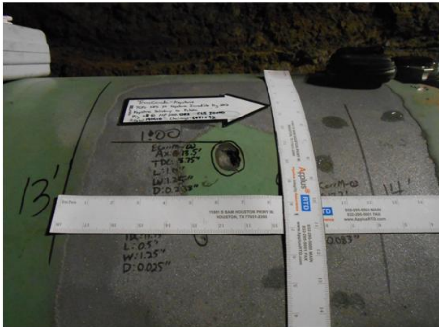
Figure 15. MP 1000.08 –External Corrosion Pitting
