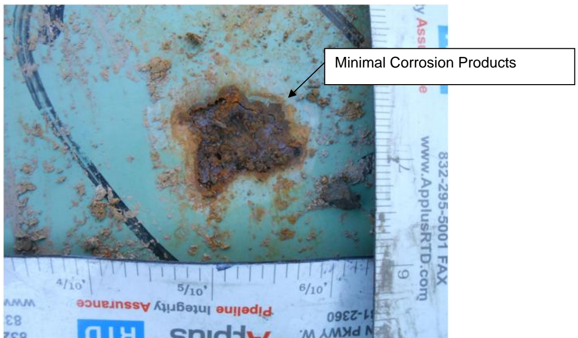
Figure 12. MP 996.33 –External Corrosion Pitting
