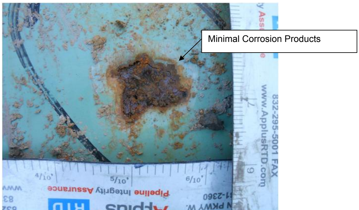
Figure 12. MP 996.33 –External Corrosion Pitting
