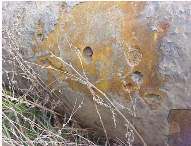
Figure 5. Typical D-C Stray Current Corrosion Morphology
