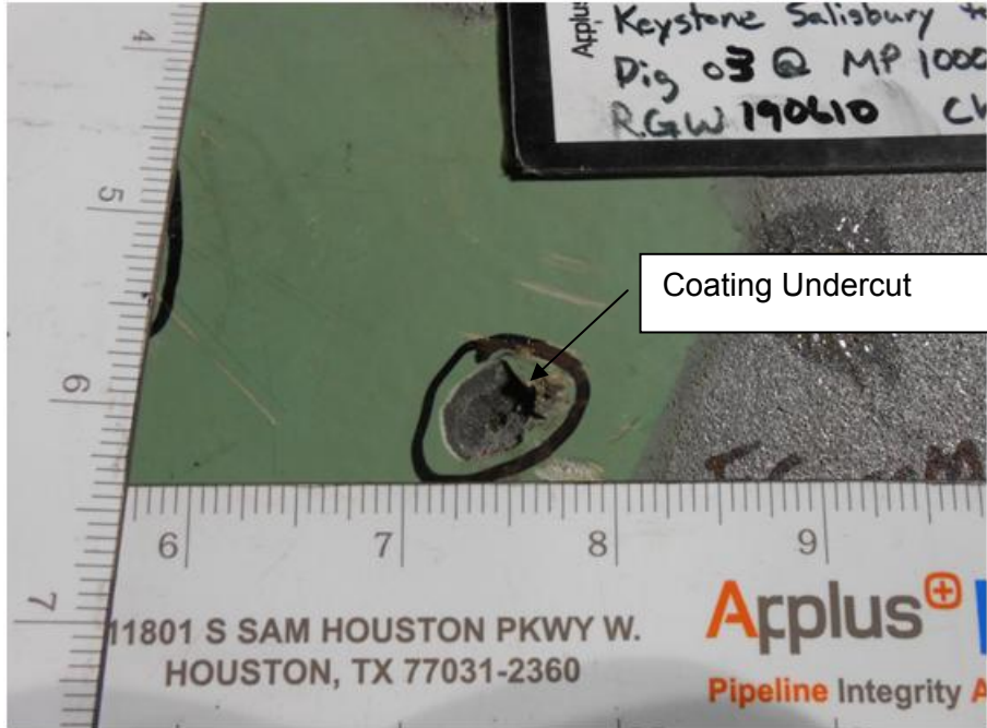
Figure 14. MP 1000.08 –External Corrosion Pitting
